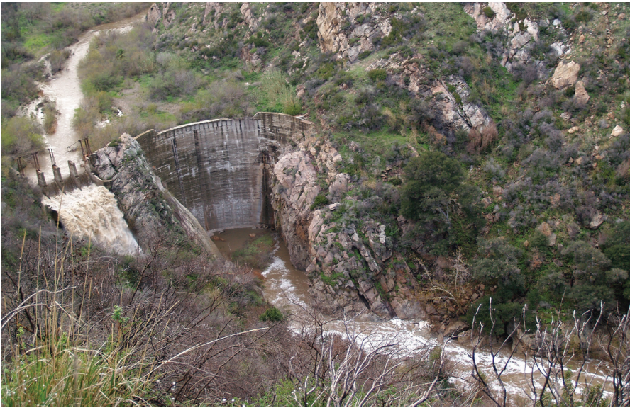
Rindge Dam on Malibu Creek, completely filled with sediment, is slated for removal so that Steelhead trout can access Upper Malibu Creek.
